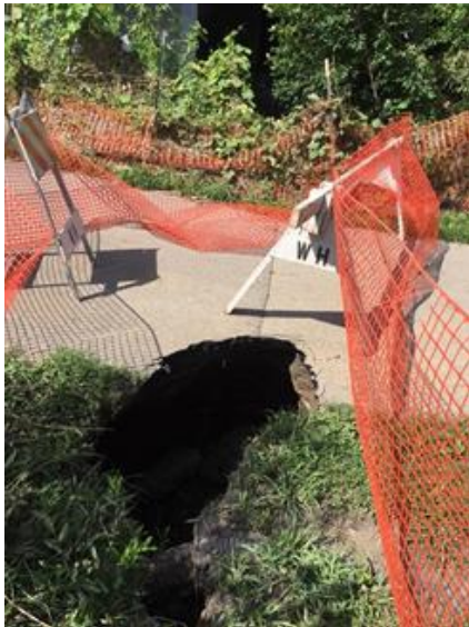
Figure 3.93.1 Windsor Heights 2018 Bike Trail Sinkhole. Source: City of Windsor Heights
