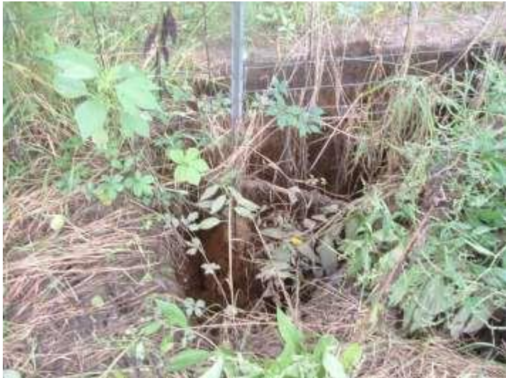
Figure 3.94. Photo of Sinkhole Near Runnells, July 28, 2010
